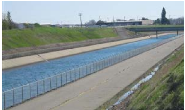
Security fencing along Folsom South Canal.
